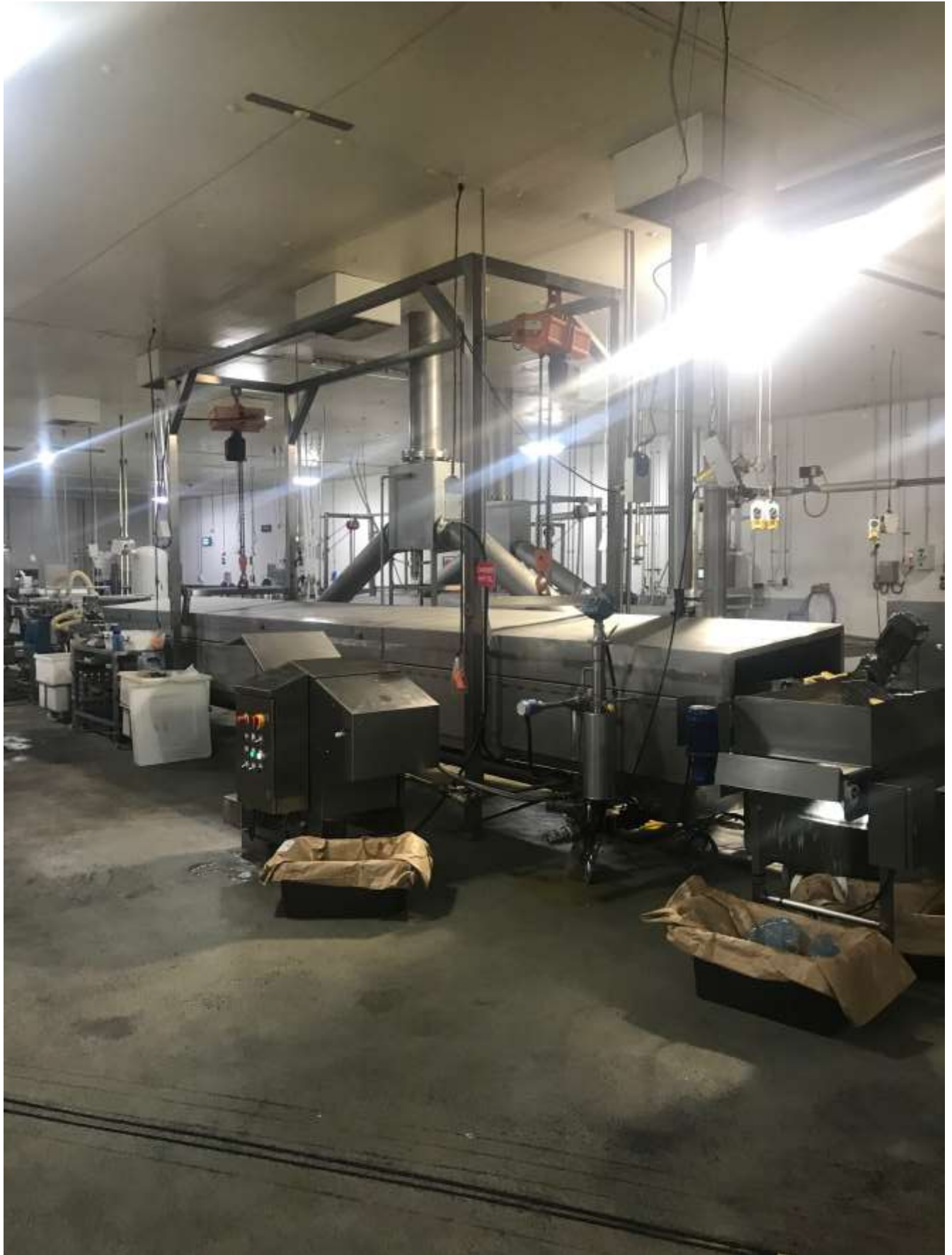
New main switchboard and MCC. Automate continuous frying system.
