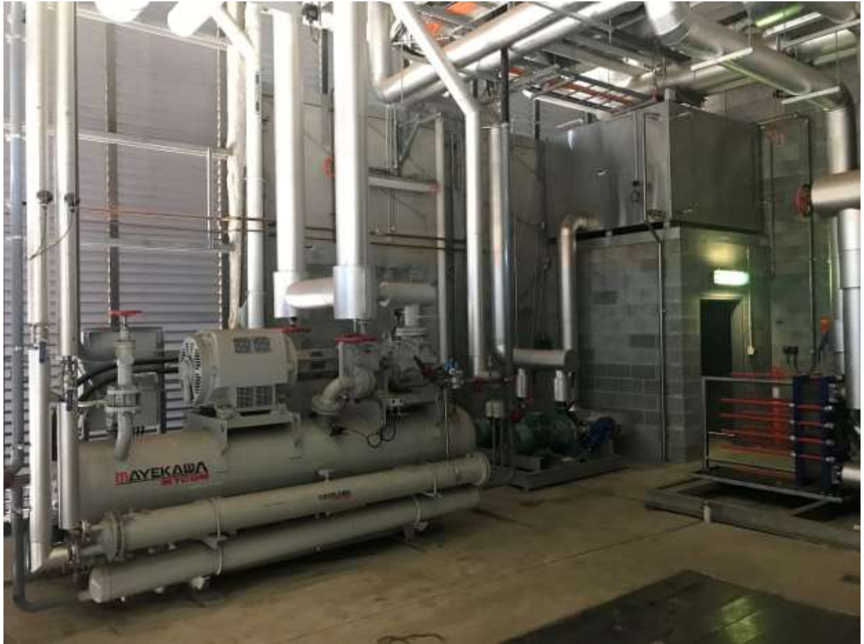
New ammonia refrigeration system plant room.
