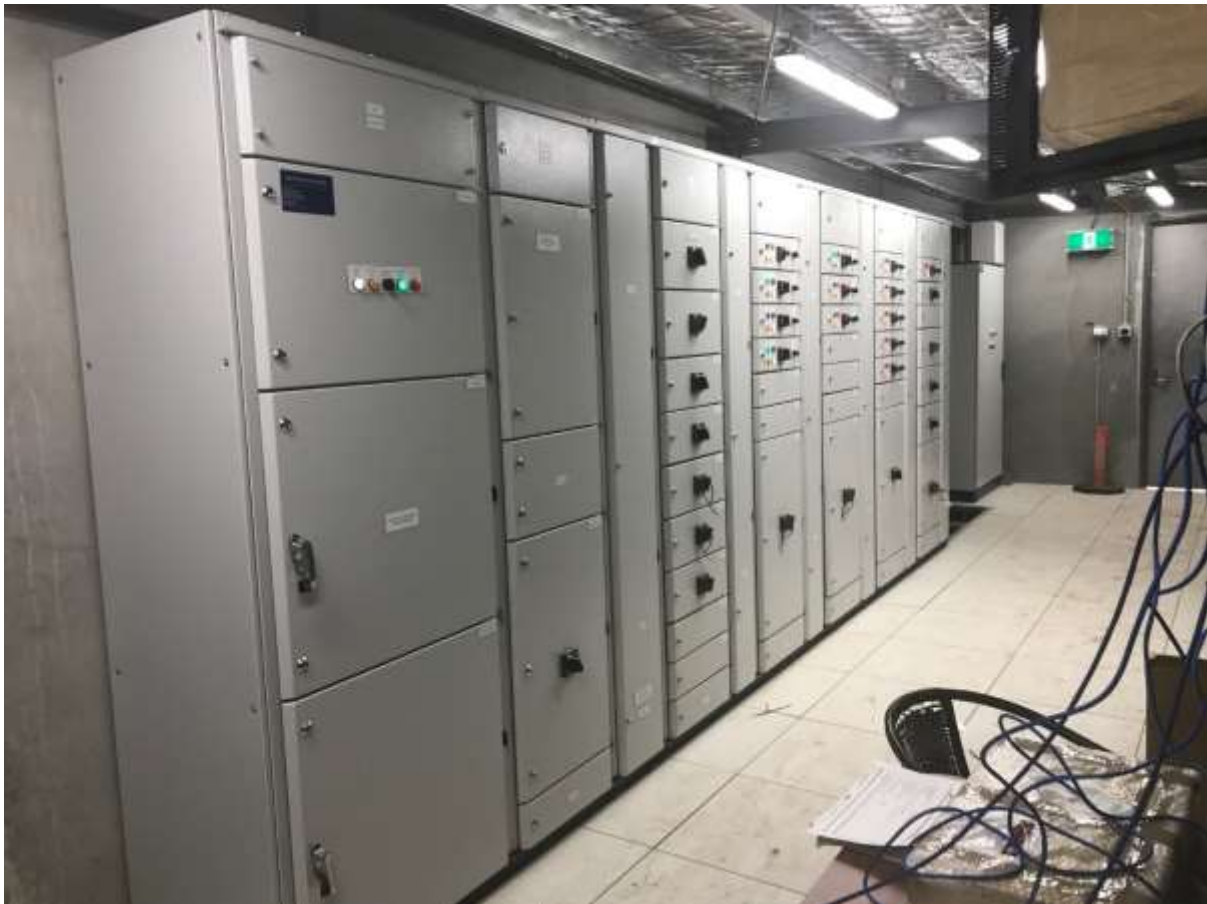
New Main Switchboard.
