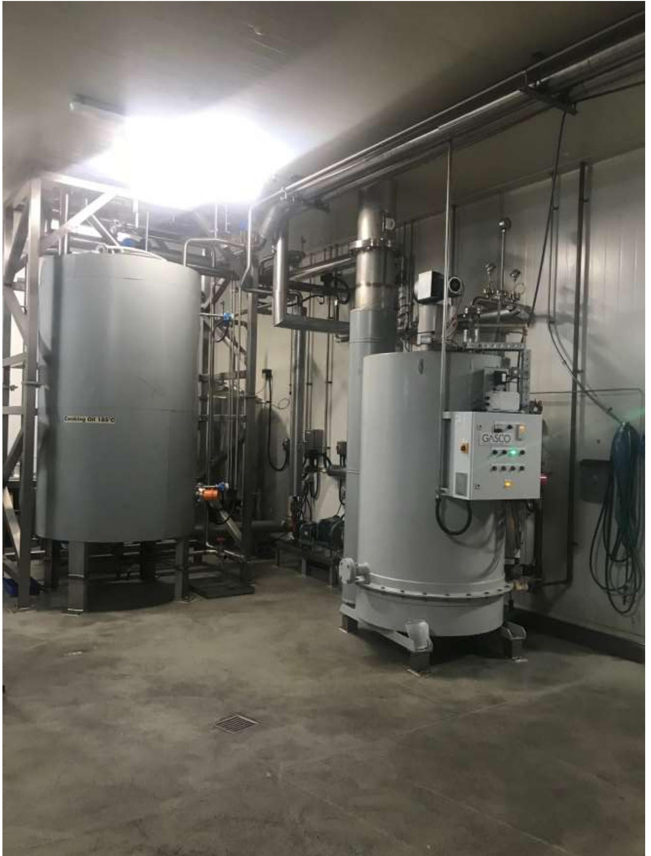
Automated Oil heating system.
